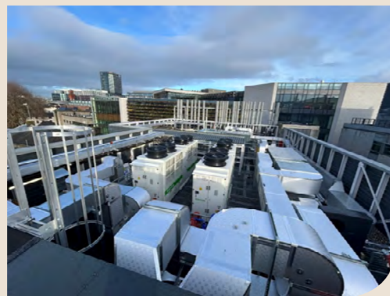
Figure 43: New Air Handling Units after Retrofit
