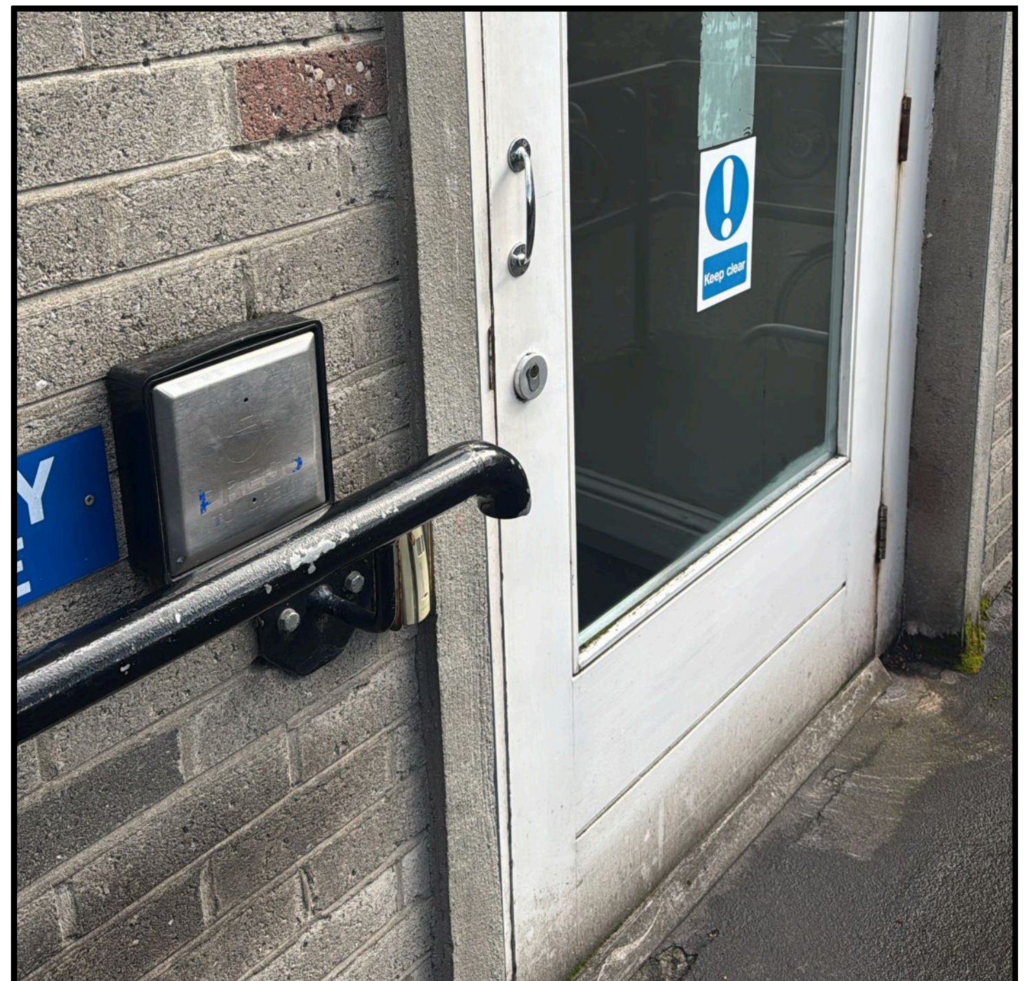
Figure 12 - Door access button obstructed by grab rail, preventing easy and intuitive use.
