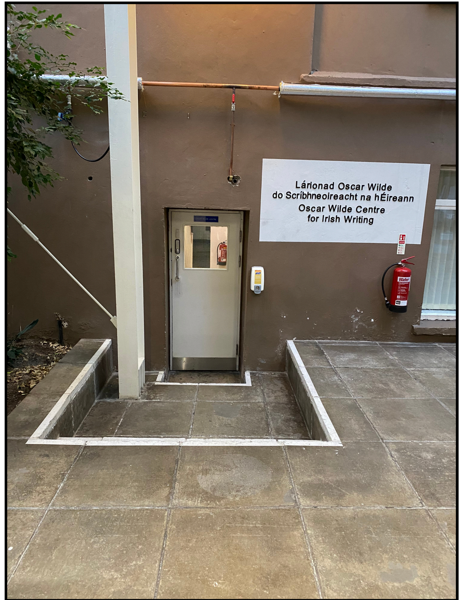
Figure 18 - Oscar Wilde Centre Entrance, located in the Hamilton Building, with steps and a separate access route, demonstrating a lack of integrated, inclusive design.
