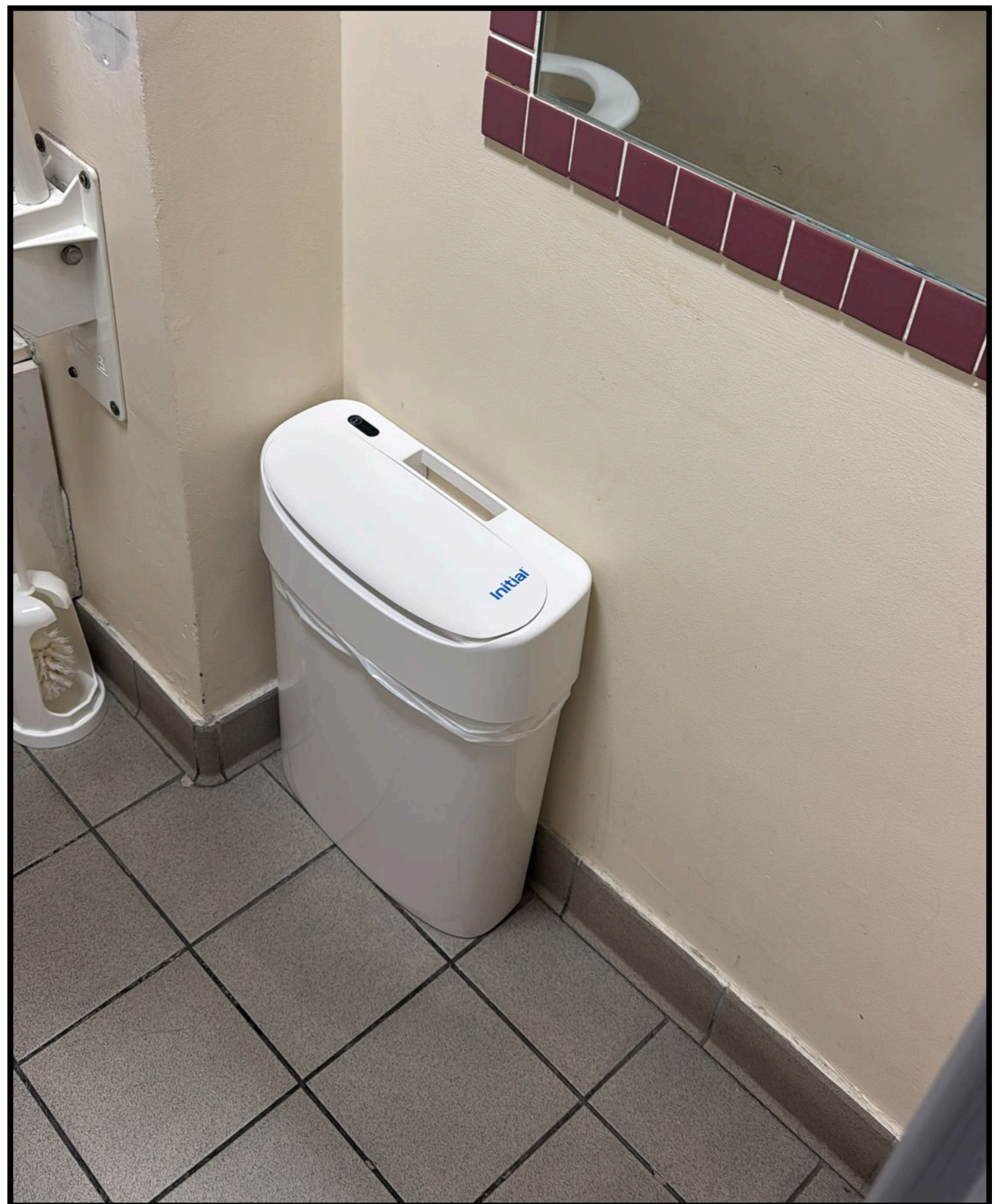
Figure 28 - Example of sanitary bin obstructing wheelchair manoeuvring space, reducing usability and independent access.
